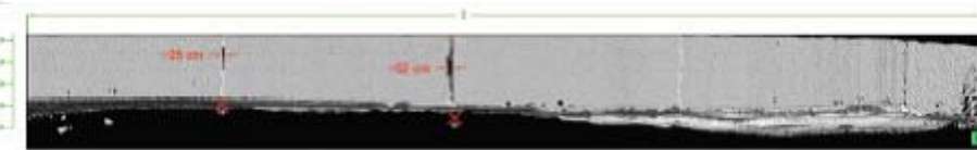
DETAILS OF CAISSON DAMAGE
